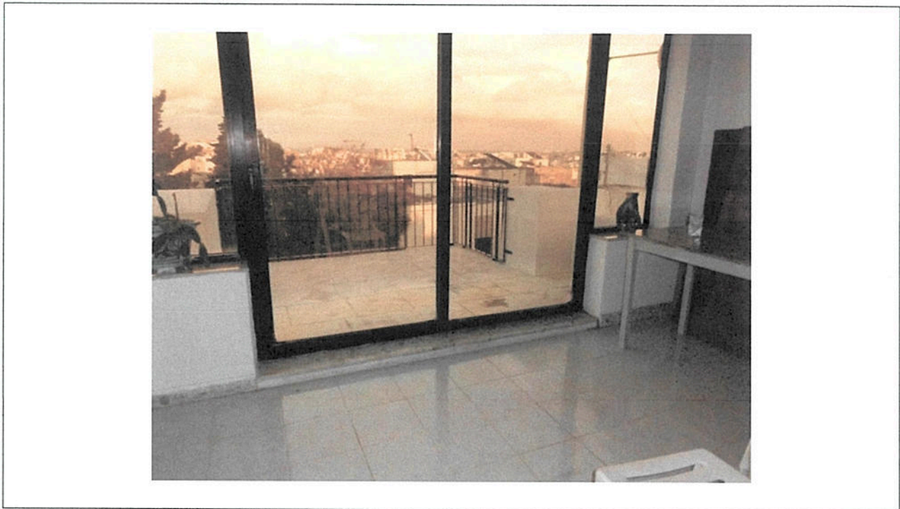
Photo 5: Photo of difference in level from outside to inside. Removal of the door sill will necessitate the disruption to the whole roof terrace
