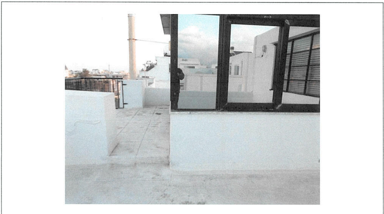
Photo 2: Note 1m high wall, which extends inside the roof build up, up to the roof's structural slab.
