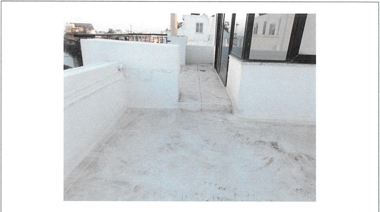
Photo 3: Existing Roof – note the disruption that will occur to the slightly elevated roof terrace, together to the waterproofed cement screed on the side roof.
